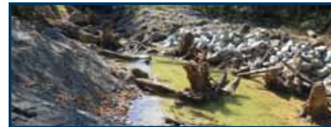
Initial restoration work through the addition of large woody debris lays the groundwork for creating refuge habitat in the channel.
